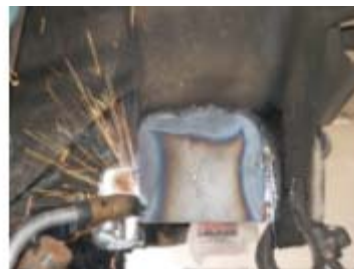
An included frame-reinforcement plate is welded over the newly exposed frame horn. After the metal cools, a coat of black spray paint helps inhibit rust.
