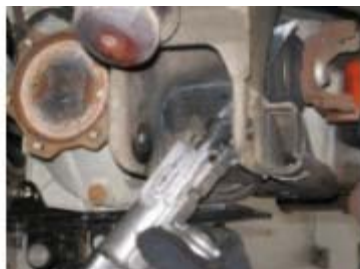
The front suspension, axles, brakes and differential must be removed. Modifications begin by trimming the driver's side diff mount. 4Wheel Parts uses a reciprocating saw.
